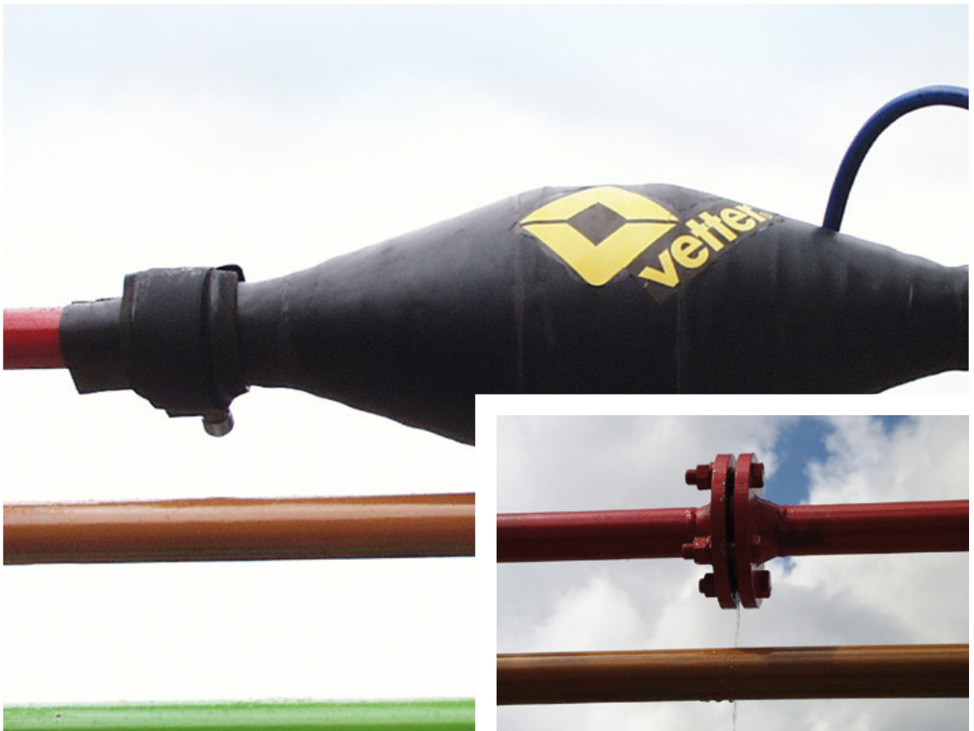
Leak in a pipe flange
